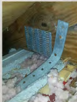
Misaligned strap greater than 1/2" gap
